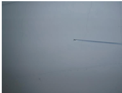
Fig. 5. Site 2: cracks in the deck underside viewed from level –2
