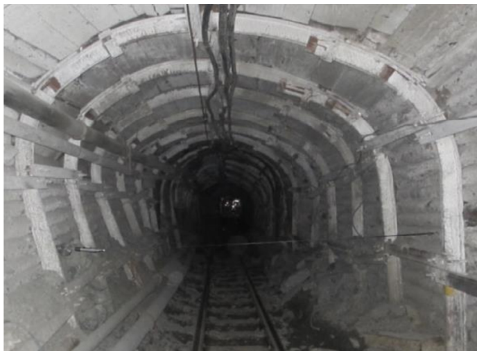
Fig. 2. Failure condition of the main haulage roadway
