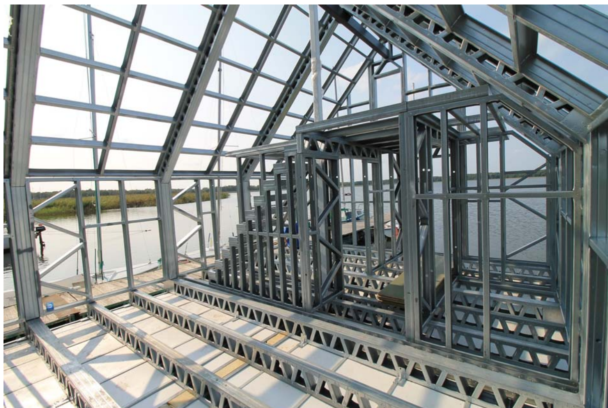
Fig. 5. Scottsdale Construction System structure raised on the steel and styrofoam platform before insulating; source: own elaboration
