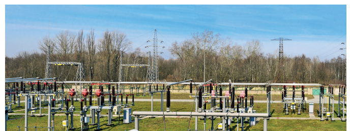
Fig. 3. Example view of the power grid object – substation
