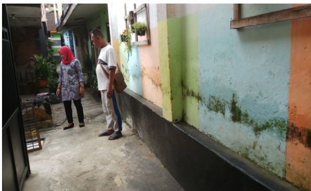
Photo 1. Flood mark at the Glintung Water Street (phot. L. Sedyowati)
