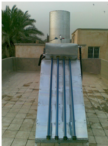
Figure 1: The evacuated tube heat pipe solar water heating system.
