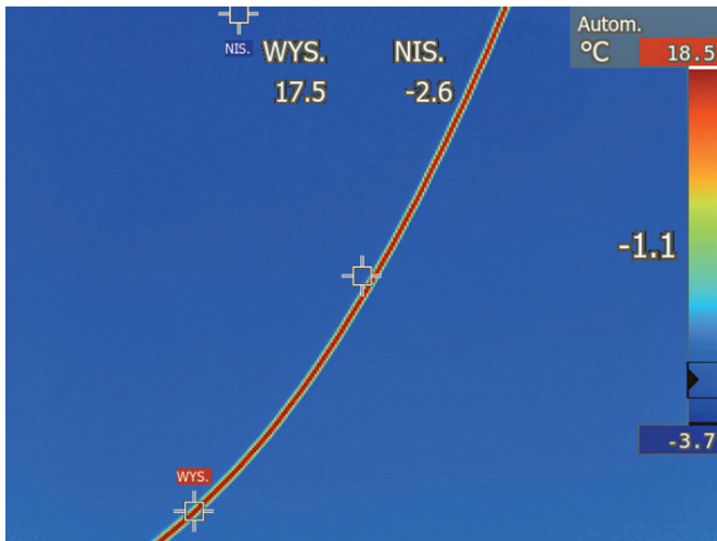
Fig. 10. Thermal image of the conductor at 9.30 p.m. Conductor temperature 17.5°C. Ambient temperature 8.5°C. Current 90 A
