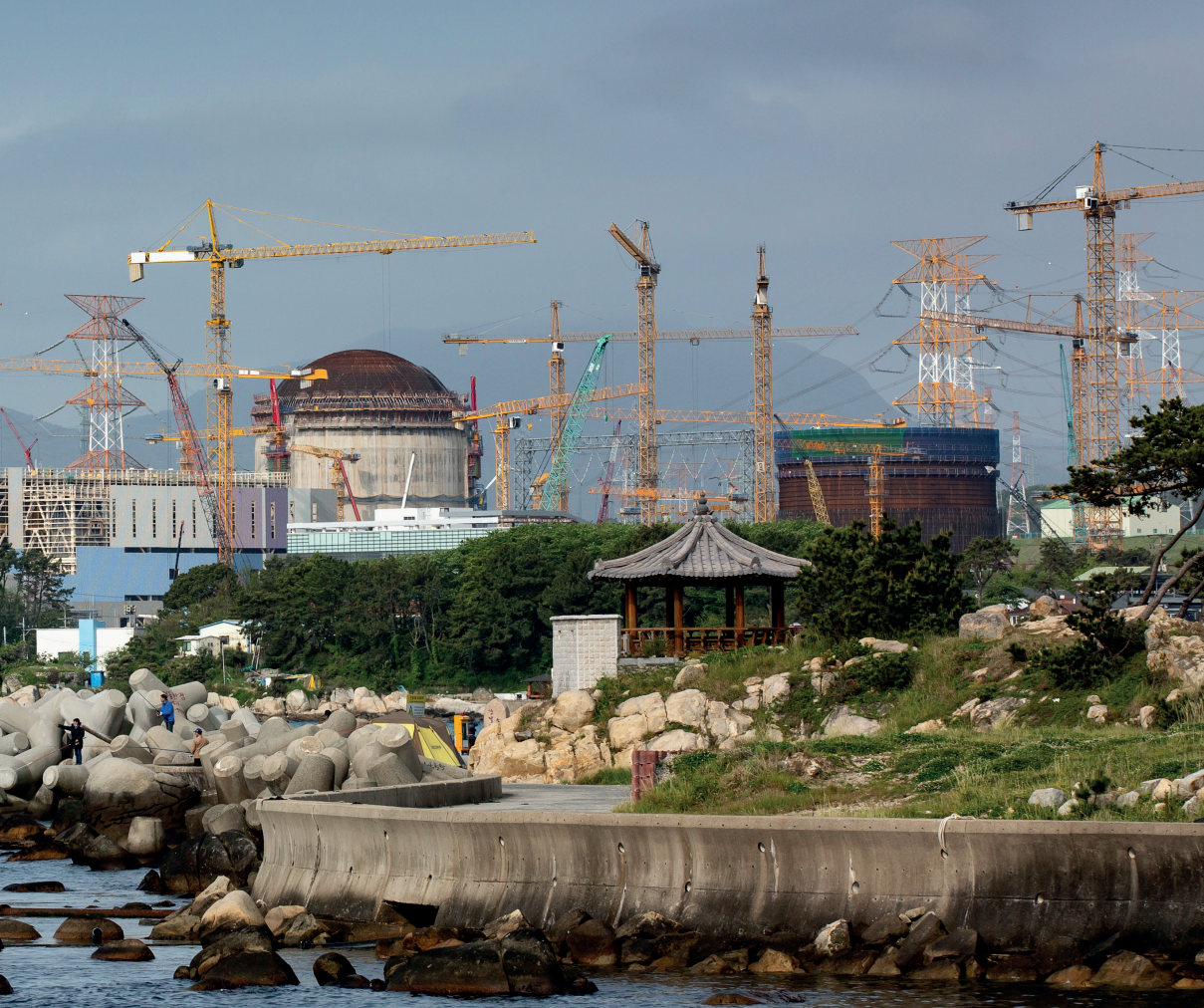
Nuclear power plant in Ulju-gun, South Korea, May 2020
