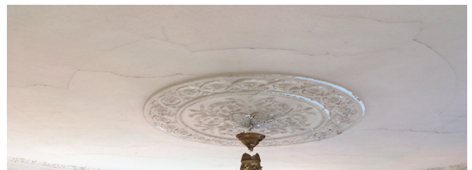
Fig. 6. Stucco on the ceiling (visible cracks in the plaster)
