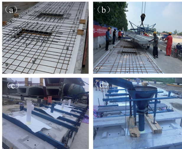
Fig. 16. The main construction steps of filling layer for CRTS III slab ballastless track; (a) Place geotextile layer and reinforced mesh; (b) Place prefabricated slab on the base plate at the presetting position; (c) Install formwork and clamps; (d) Cast concrete from the top pouring hole
