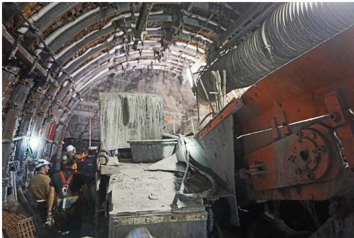
Fig. 1. View of the mining face of a gallery drilled with a roadheader
