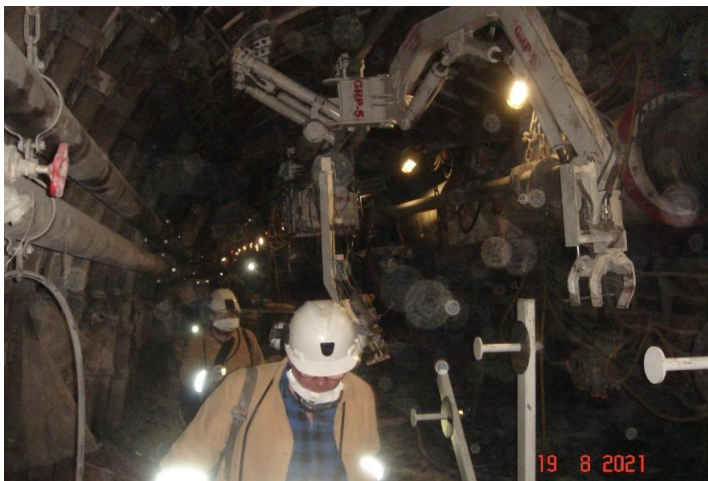
Fig. 18. View of the MZT-M installed in an underground excavation
