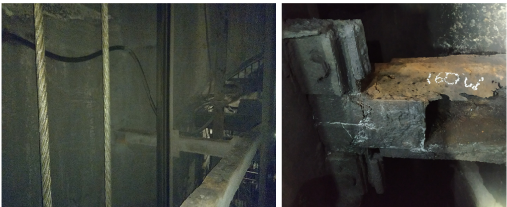
Fig. 3. Corrosion in a mine shaft
