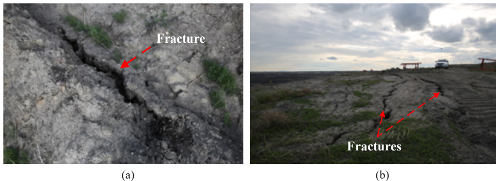
Fig. 7. Fractures appeared on the surface of the transportation bench. (a) Induced fractures at the 920 m level. (b) induced fractures and slope deformation at the 944 m level
