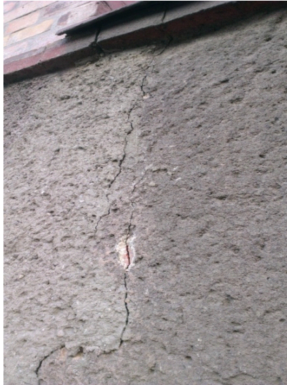
Fig. 12. Vertical cracking in the central part of the facade wall of Building A ( source: own work )
