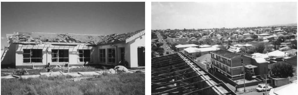
Fig. 19. Substantial damage in South Africa.
