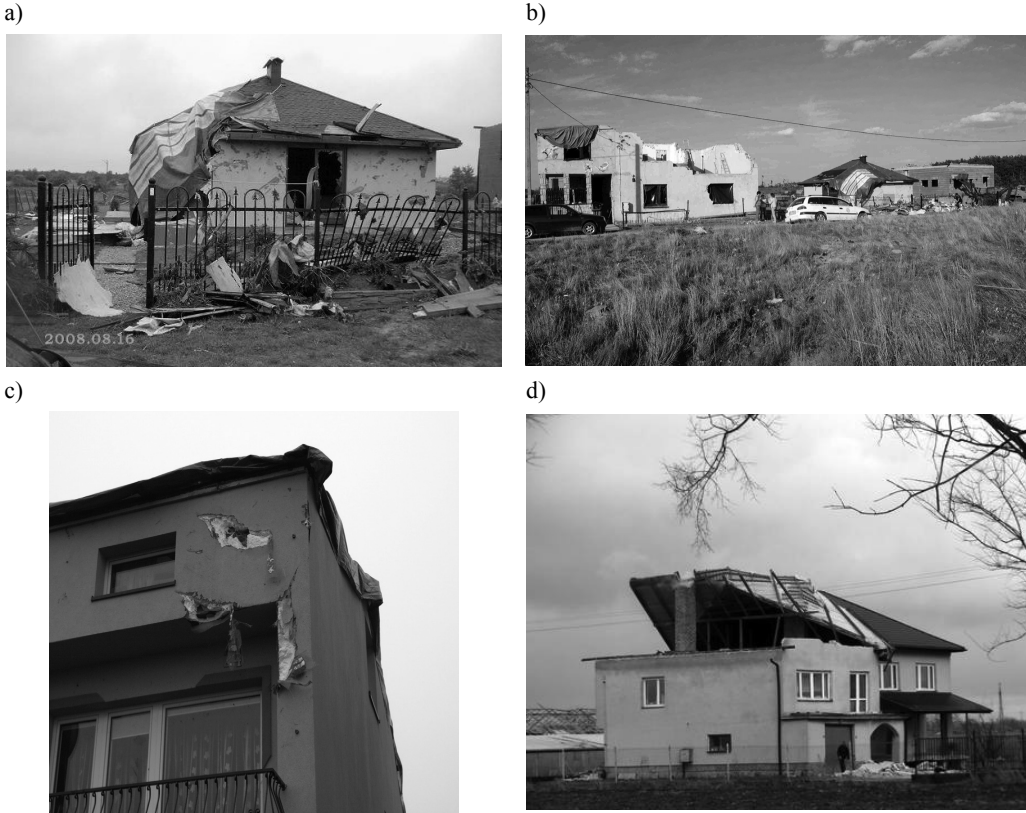
Fig. 17. Typical examples of damage to houses caused by tornadoes in Poland; a) damage to the building of frame construction, b) partial removal of the 2nd storey of a building (Phot. G. Beblot), c) damage to walls inflicted by windborne debris, d) failure of a sheet metal roof.
