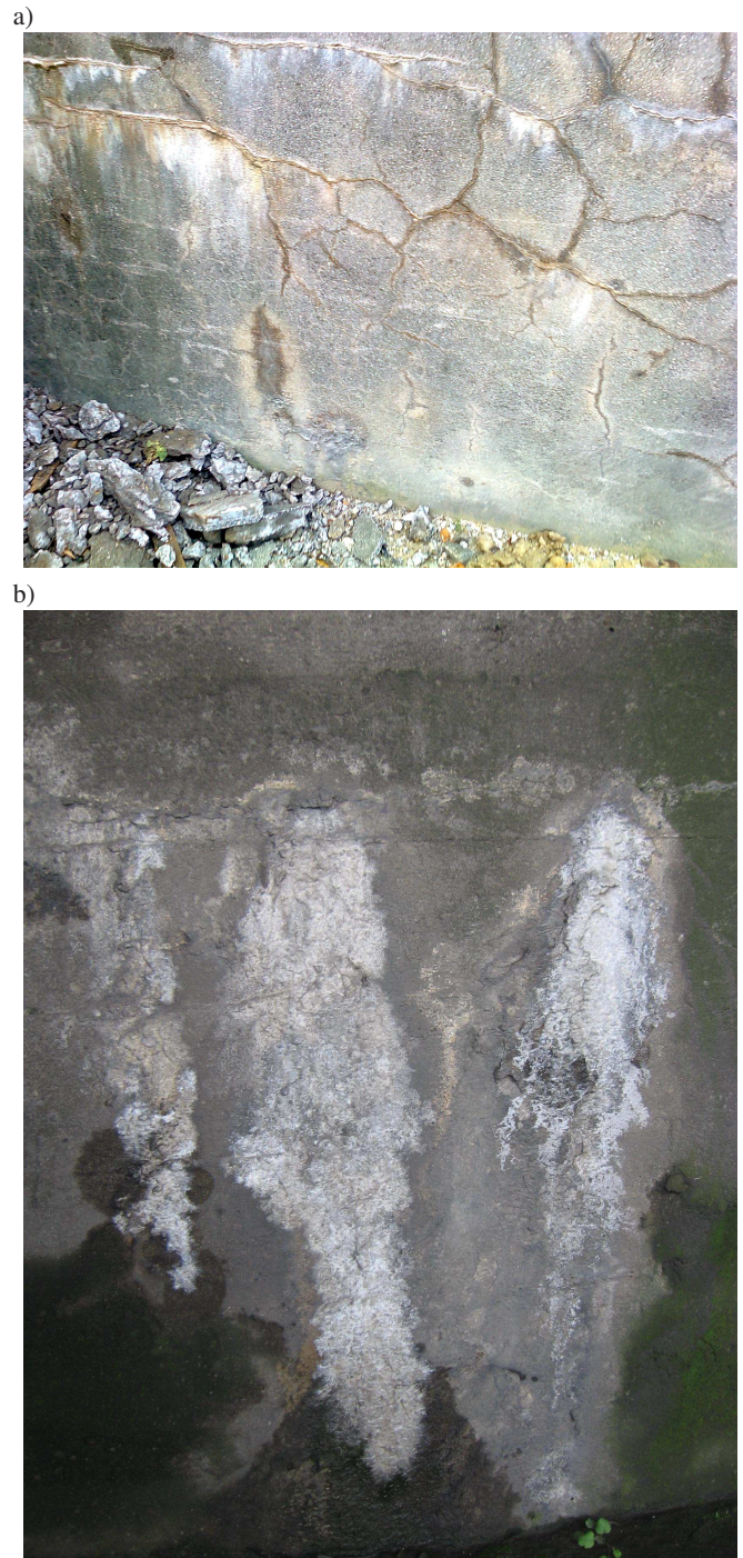
Fig. 4. a) Flyover pier with ASR symptoms, b) gel exuding on the surface of concrete
