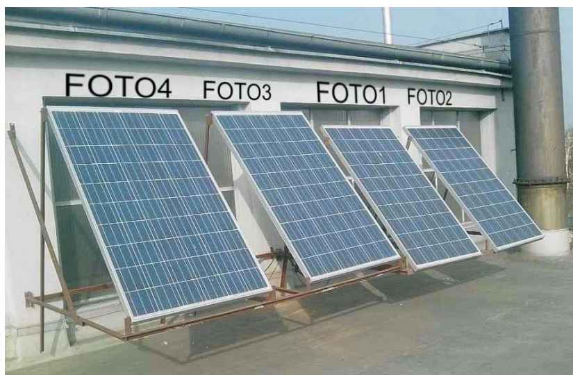
Figure 2. The photovoltaic panels IBC-225TE.
