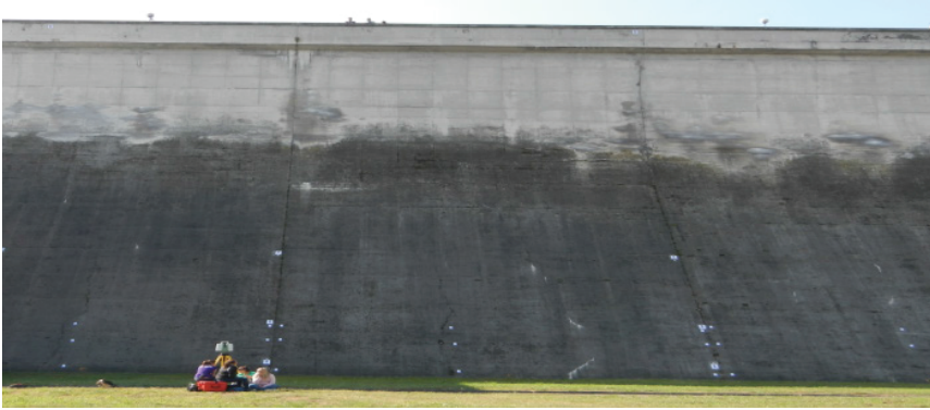
Fig. 5. Optical photo of the fragment of the tested concrete wall
