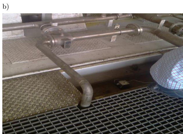
Fig. 14. Locations of the vibration measurement on the foundation of the CO 2 compressor: a) position F1, b) position F2.
