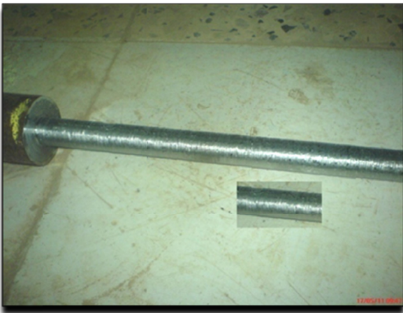
Fig. 9. Poor surface finish
