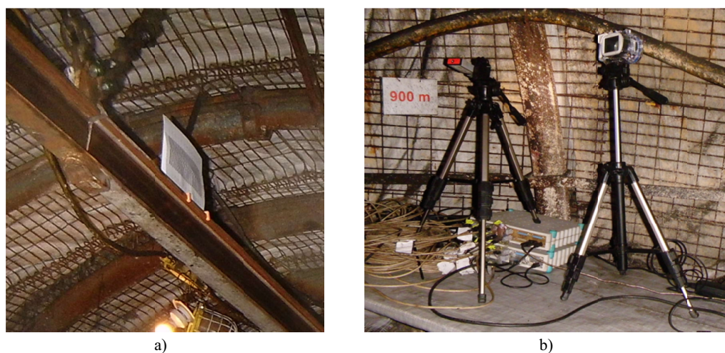
Fig. 8. The measuring stand for the suspended route displacement: a) scale mounted on the upper part of the I155 beam, b) measuring station
