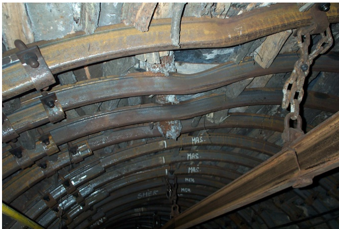
Fig. 7. Buckled roof arches
