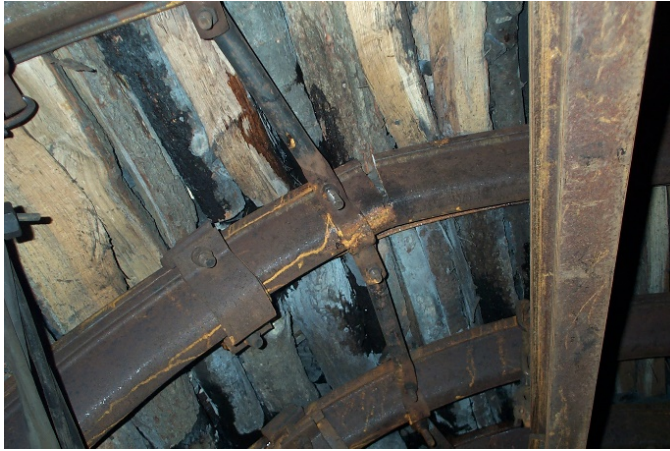
Fig. 6. Roof arch fracture
