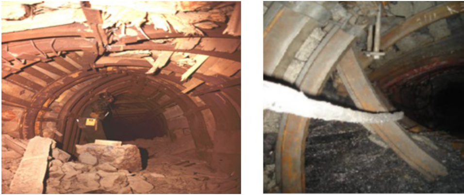
Fig. 2. Loss of stability of underground workings in the Cam Pha coal basin
