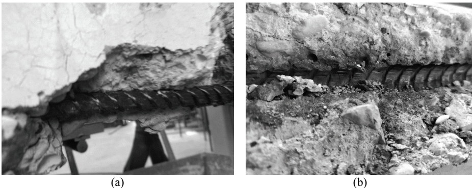
Fig. 7. De-bonding of HFRP bars: (a) separated HFRP bars after being uncovered from concrete; (b) concrete surface after taking the bars out.
