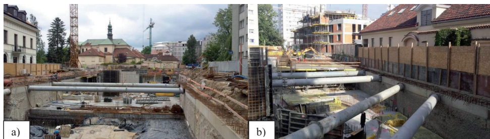
Fig. 2. Implementation of the underground building complex a) construction of the foundation slab, b) construction of the walls and pillars of the underground storey.
