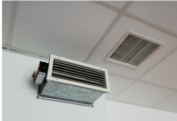
Fig. 4. View of the air-conditioning outlet.
