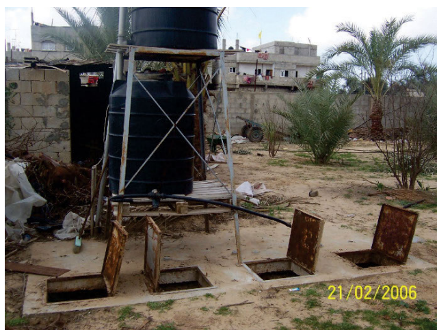
Photo 1. Graywater system used by the Palestinian Agricultural Development Association in Palestine along with the openings of each treatment chamber (phot.: R. Alkhatib)
