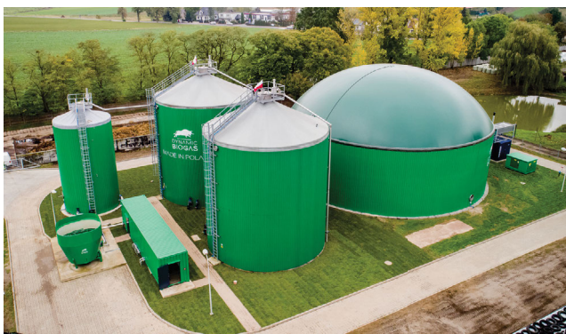
Photo 3. 0.5 MWe biogas plant (Dynamic Biogas technology) with separated acid hydrolysis built in PULS experimental farm in Przybroda in 2019 (phot.: J. Dach)
