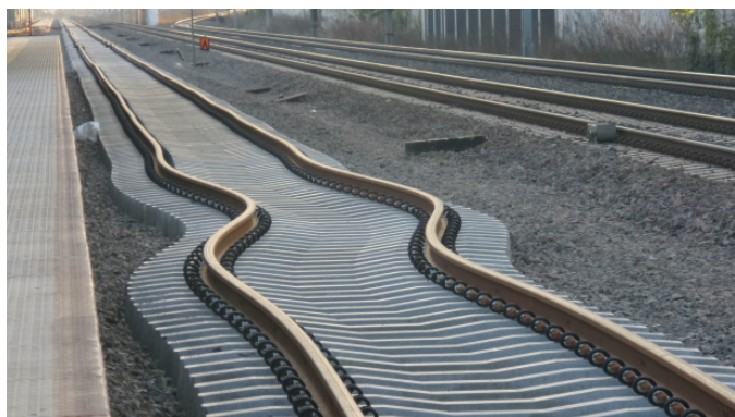
Fig. 1. Contactless track buckling [8]
