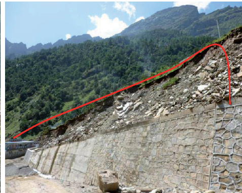
Fig. 5. Back wall of the landslide
