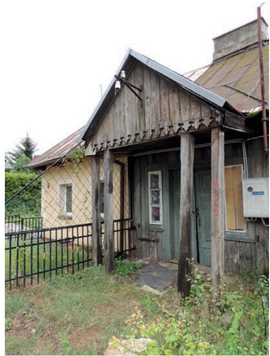
Ill. 5. Detail of the house at 8 Podzamcze Street in Hrubieszów. Photo by B. Makowska, 2022.
