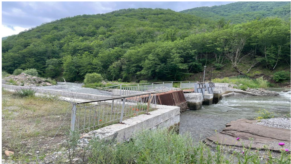
Fig. 2. Water intake structure for small hydroelectric power plants Source: developed by the author
