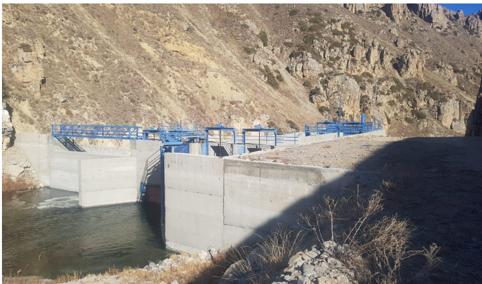
Fig. 3. Water intake structure for small hydroelectric power plants Source: developed by the author
