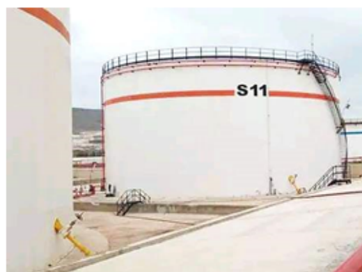
Fig. 3. Diesel storage tank S11
