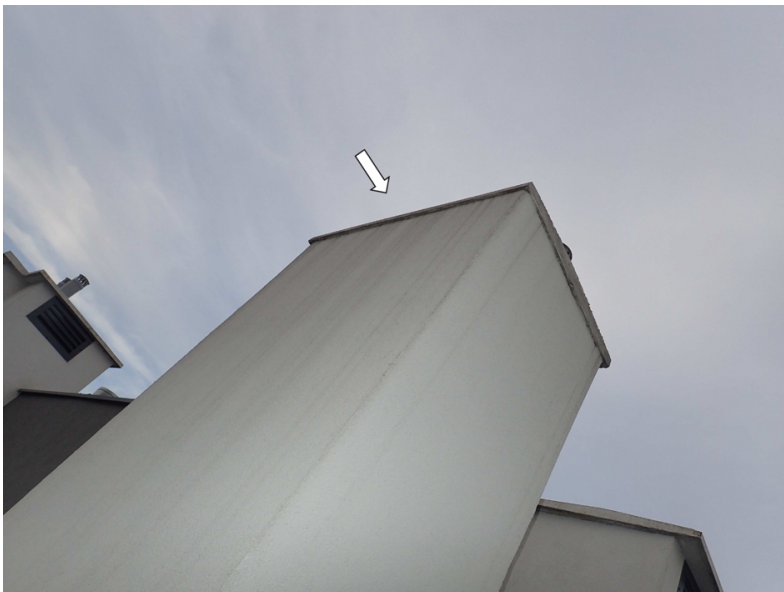
Fig. 2. Chimney caps with too small a drip causing stains on the chimney shaft
