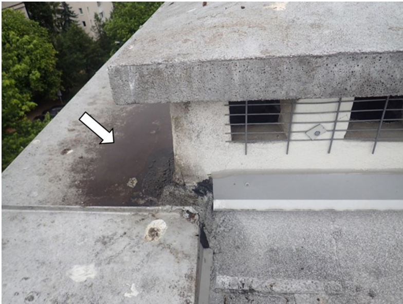
Fig. 1. Steel flashing of the attic at the chimney made in a way that prevents water from flowing out. There was moisture on the façade below
