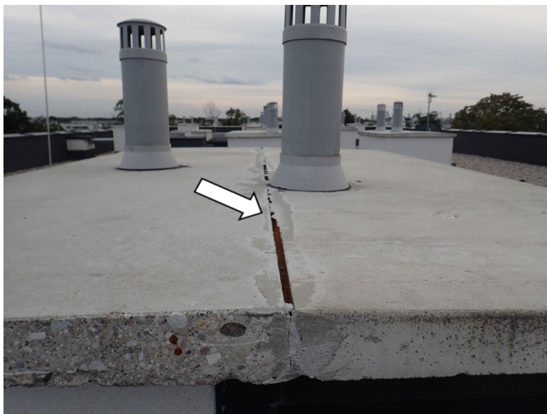
Fig. 3. The chimney cap is made of two prefabricated concrete slabs. Plates are not connected to each other, which let water inside the chimney
