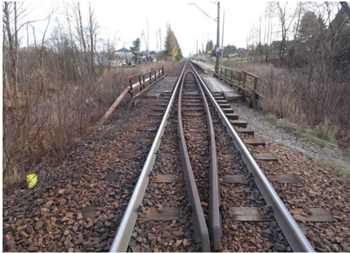
Fig. 10. Loss of ballast on the bridge approach
