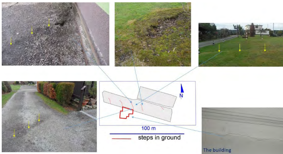
Fig. 3. View of discontinuous linear deformations formed in years 2015–2021
