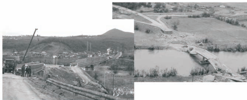
Fig. 10. Bridge failure and its reconstruction using fold-up segments.
