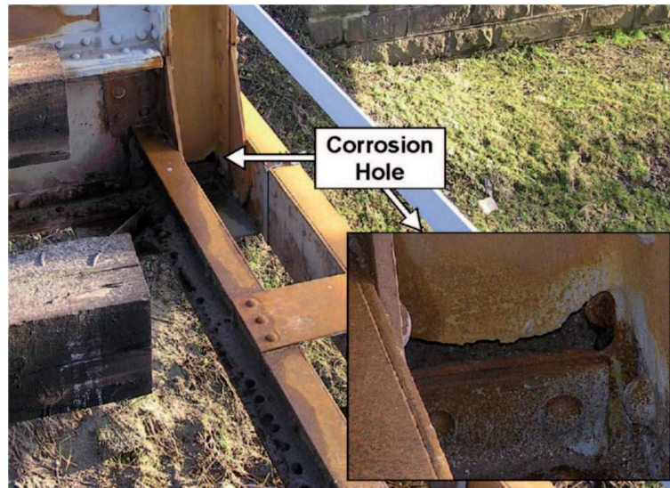
Fig. 1. Damage due to corrosion in structural element of a bridge.
