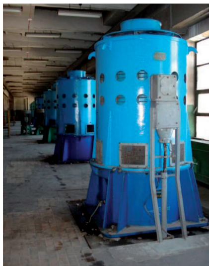
Fig. 1. Electric engine of the pump
