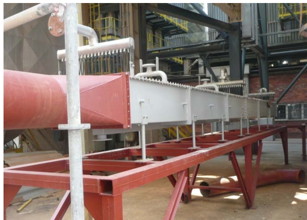
Fig. 7. Pilot scale 312 kW condensing heat exchanger in PGE Belchatów power plant
