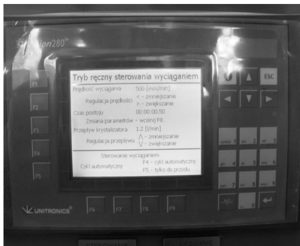
Fig. 2. View of control panel
