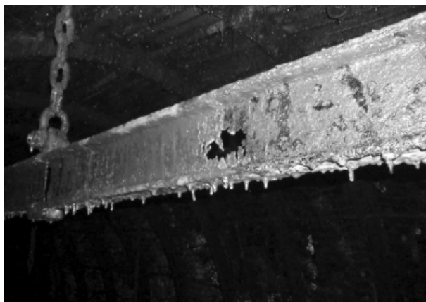
Fig. 1. Accelerated degradation of the lifting beam in coal mine environment (steel 3)
